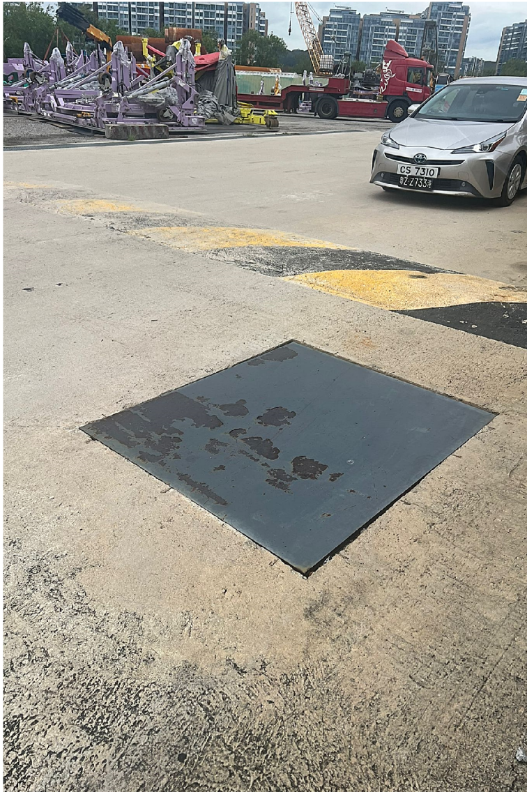
Photo 1 showing Ex. MH A1
